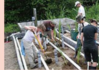
Staff from Fleming's Centre for Alternative Wastewater Treatment completing a research project.
