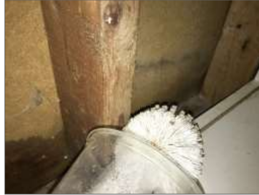
Photo 6 - Mould growth on wood fibre panel identified in closet area
