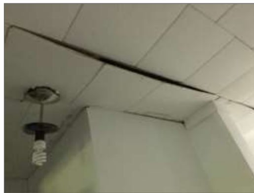
Photo 2 - Ceiling falling in, in corridor of Cabin.
