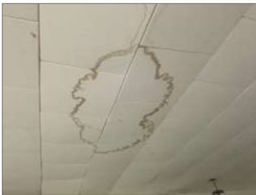
Photo 1 - Typical water staining identified on 1x1 tiles in various locations throughout the cabin.
