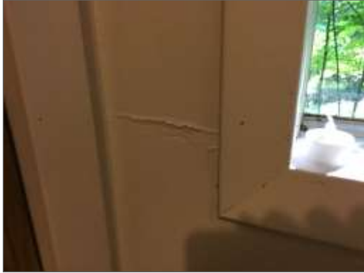
Photo 3 - Cracks in drywall could be due to building shift or past water infiltration.
