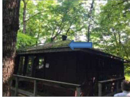
Photo 4 - Organic growth on Cabin roof
