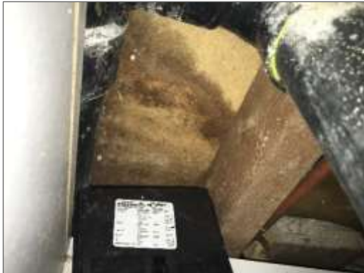
Photo 7 - Mould growth on wood fibre panel behind kitchen sink drywall that was replaced.
