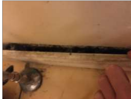
Photo 8 - Mould growth behind loose baseboard in washroom.
