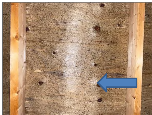
Photo 19 - Typical spotting observed on side walls of attic space.
