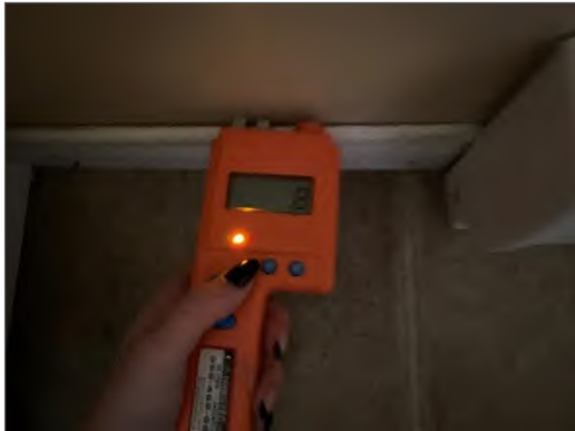
Photo 38 - Wet wall identified behind toilet.
