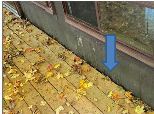
Photo 31 - Exterior wood siding is beginning to rot due to water.
