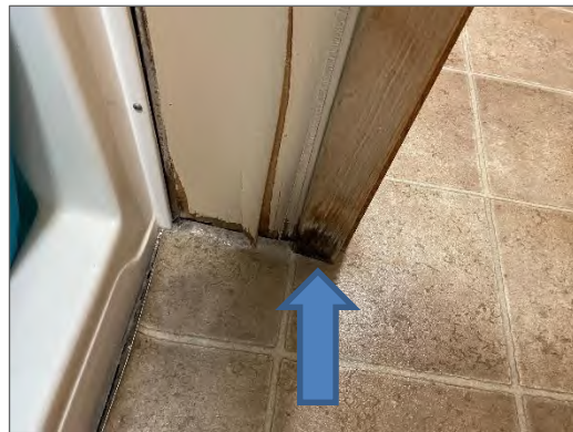
Photo 26 - Black spotting on wooden door frame and damage to wood panelling by shower confirmed mould (TL-08).
