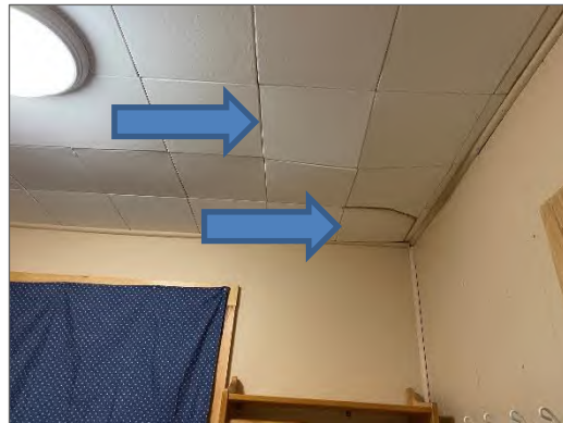
Photo 24 - Water stained ceiling tile and ceiling falling in.
