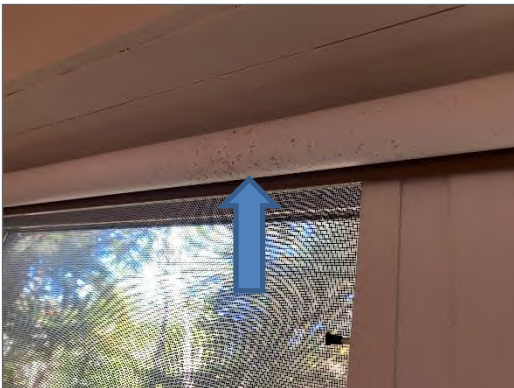
Photo 56 - Black spotting on curtain in bedroom.
