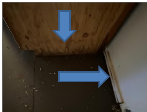
Photo 6 - Water damage on lower part of wood cabinets and slight mould growth on drywall (TL-01) where stove would go.
