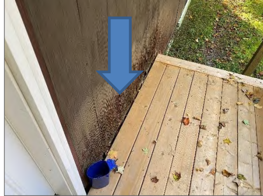
Photo 22 - Lower portion of exterior wood siding is rotting in various locations.
