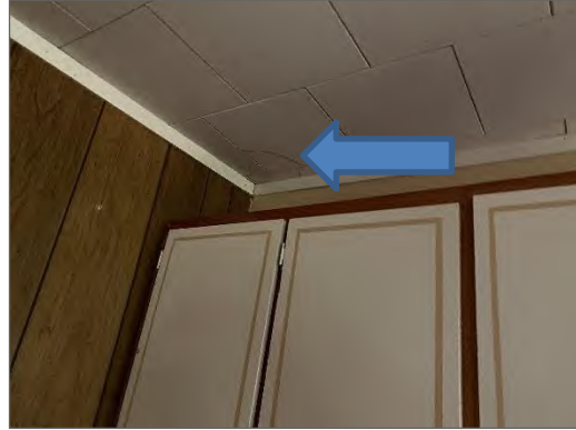
Photo 37 - Typical water stained ceiling tiles identified throughout cabin.
