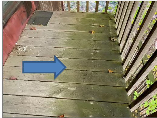
Photo 10 - Organic growth/water damage on balcony.
