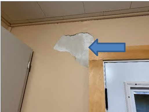
Photo 23 - Water damage by exterior door.
