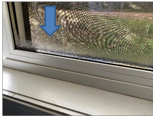
Photo 17 - Typical condensation on windows identified throughout the cabin.
