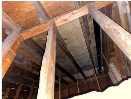
Photo 51 - No suspect mould identified in attic space.
