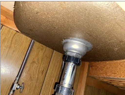
Photo 32 - Asbestos containing sink mastic on sink in Kitchen.
