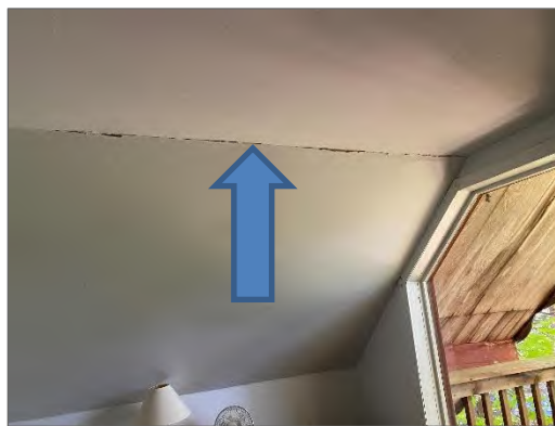
Photo 13 - Cracks in drywall due to building shift.
