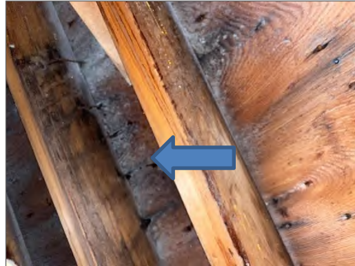
Photo 28 - Spotting identified on wood in attic space on all sides.
