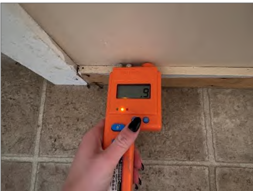
Photo 34 - Wet wall adjacent to exterior door.
