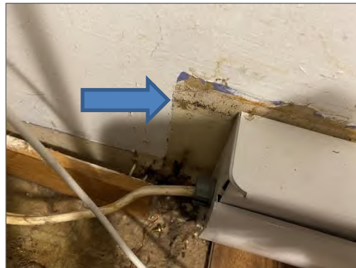
Photo 48 - Black spotting behind radiator in Closet confirmed mould growth (TL-09).
