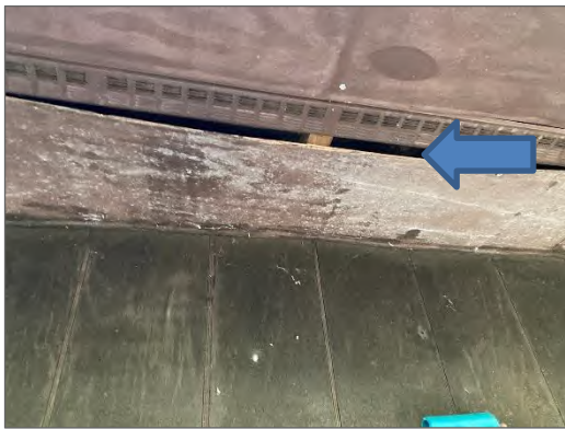
Photo 16 - Gap in underside of overhang to attic space.
