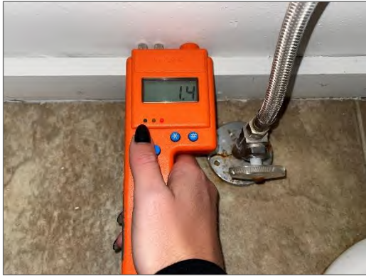
Photo 7 - Wet wall behind toilet in Washroom.
