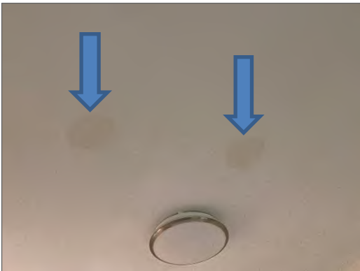
Photo 54 - Water staining on drywall ceiling in Bedroom.
