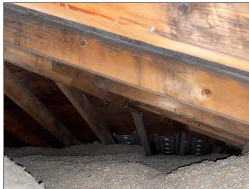
Photo 29 - Spotting identified on wood in attic space on all sides.
