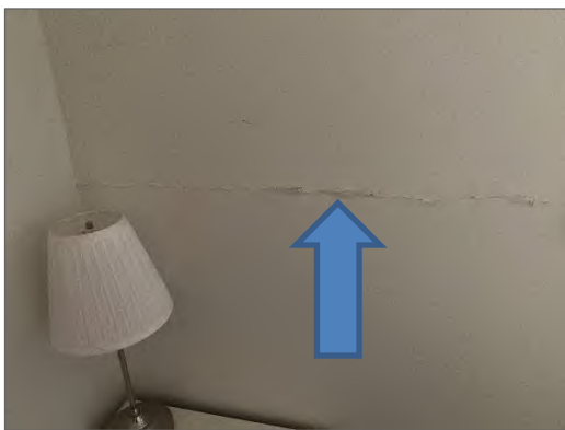
Photo 5 - Cracks in drywall walls due to building shift.
