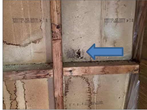
Photo 59 - Water staining and mould growth on drywall wall in Pump Room (TL-05).
