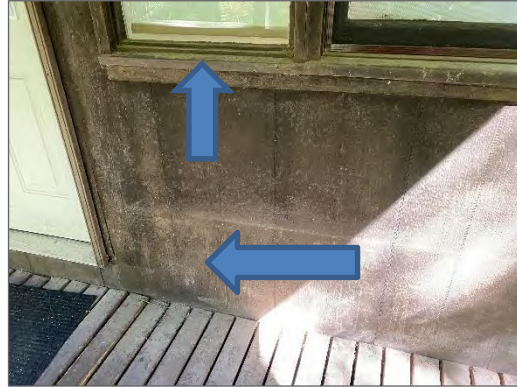
Photo 53 - Organic growth and rotting exterior siding.
