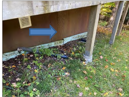
Photo 42 - Organic growth on wood siding and Styrofoam.
