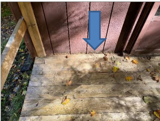
Photo 11 - Lower part of wood exterior panelling is starting to rot.
