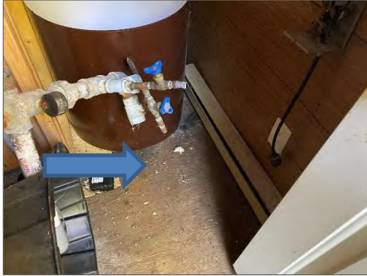
Photo 58 - Rodent droppings in Pump Room.
