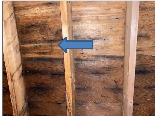
Photo 39 - Typical light spotting identified on all sides of attic.
