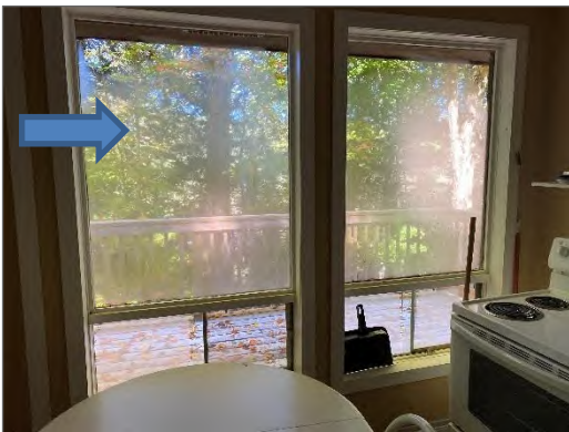
Photo 43 - Condensation on windows throughout the cabin due to poor insulation.
