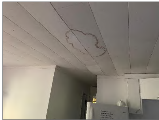
Photo 4 - Typical water staining identified on 1x1 tiles in various locations throughout the cabin.
