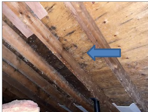
Photo 40 - Typical spotting identified on all sides of attic.
