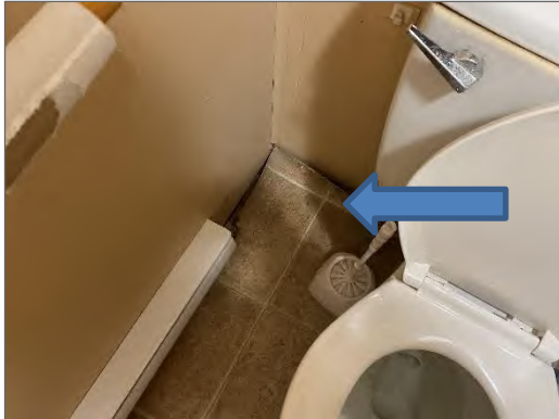
Photo 27 - Flooring by toilet is lifting due to water damage.
