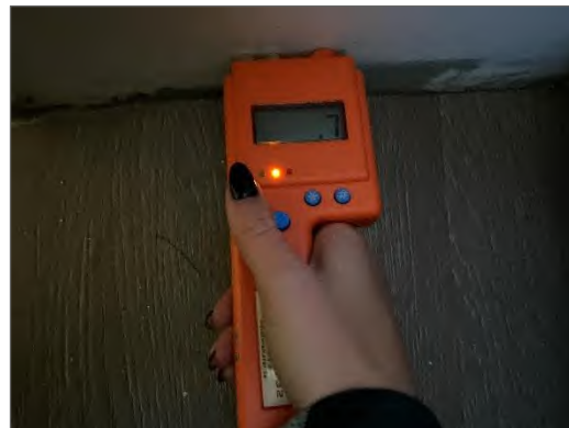
Photo 44 - Wet wall in washroom.
