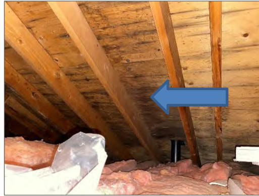
Photo 8 - Typical spotting observed in attic space.
