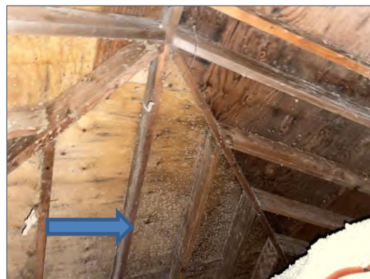
Photo 46 - Typical spotting identified on all sides of attic.
