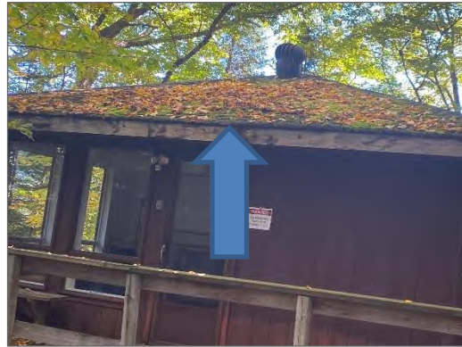
Photo 2 - Organic growth on cabin 1 roof.
