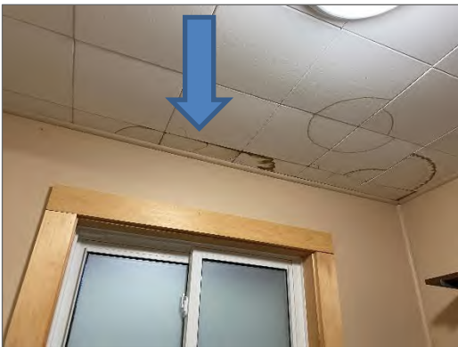
Photo 25 - Typical water stained ceiling tiles identified throughout cabin.
