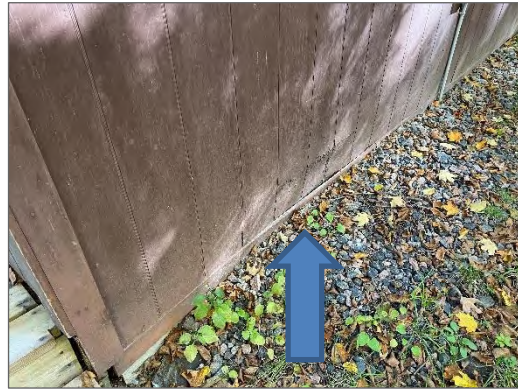
Photo 15 - Exterior wood siding is warping.
