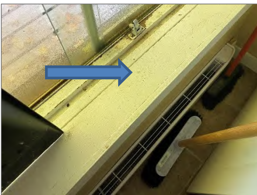
Photo 45 - Spotting identified on window frame confirmed to be mould growth (TL-04).
