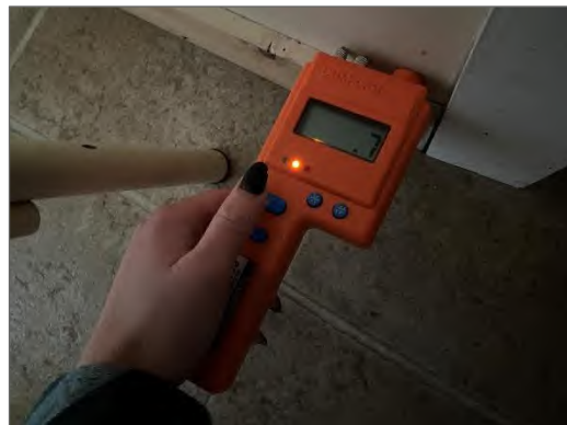
Photo 35 - Wet wall adjacent to other exterior door.
