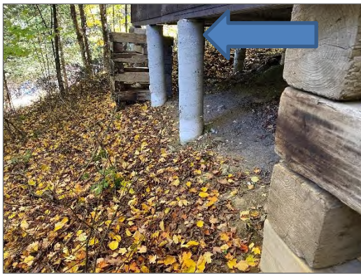
Photo 3 - Erosion on concrete cinderblocks and cabin is shifting off the blocks.
