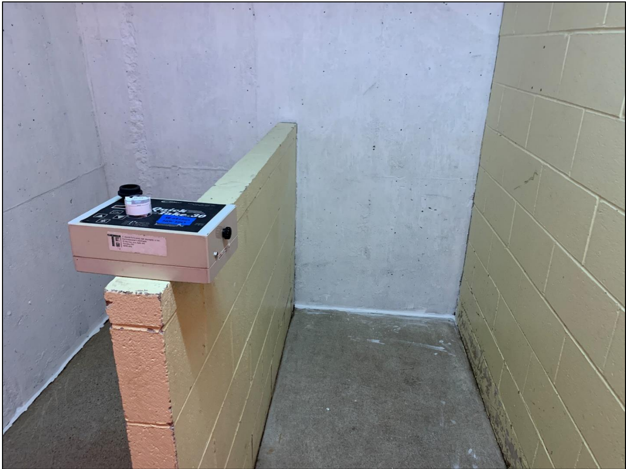
Photograph 1: View of the affected area where remediation procedures were taken for a level 2 mold contamination.
