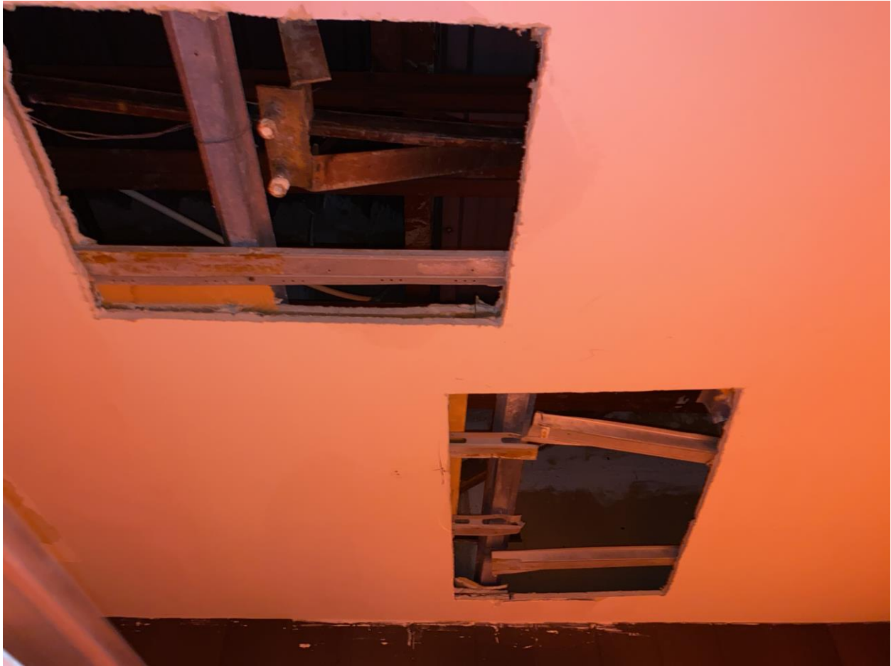
Photograph 1: View of the project area ceiling where approx. nine (9) ft 2 of asbestos-containing drywall was removed.
