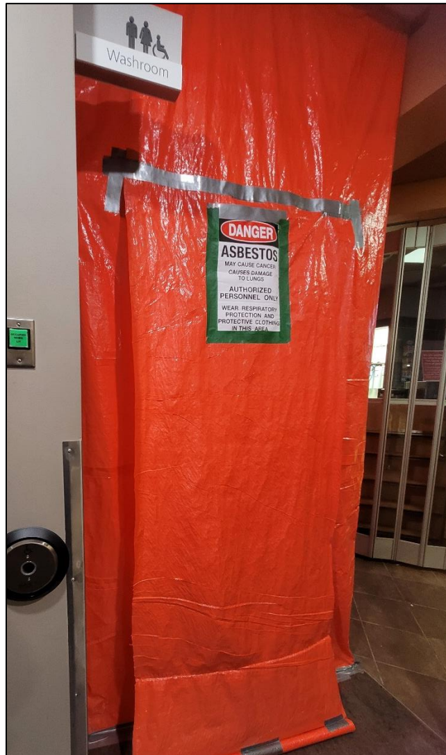
Photograph 1: View of the entrance to the enclosure where there is visible asbestos danger signage on the door.
