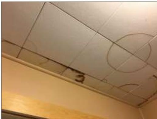
Photo 9 - Typical water staining identified on 1' x 1' tiles in various locations throughout the cabin.
