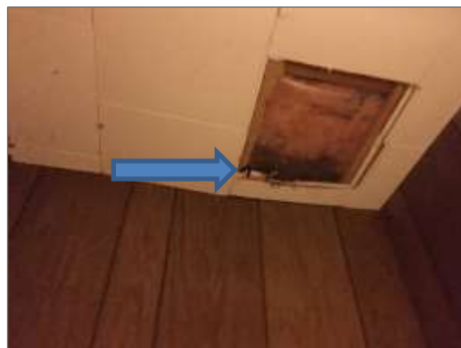
Photo 12 - Water staining identified in vapour barrier through access hatch.
