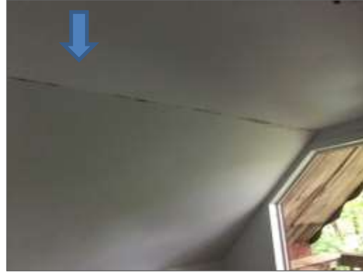
Photo 4 - Typical cracking identified in bedrooms on second floor.
