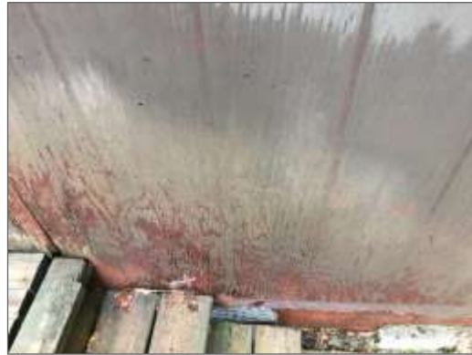
Photo 8 - Rotting wood panelling exterior of cabin.
