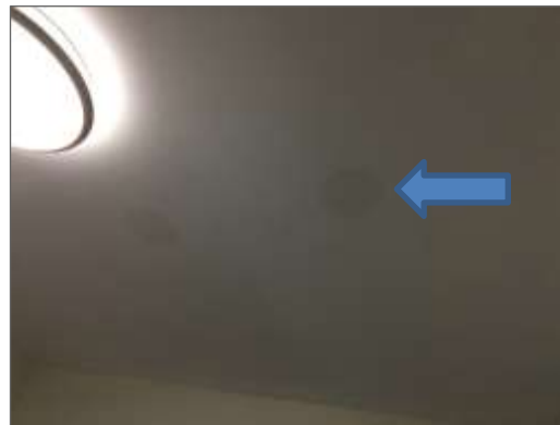
Photo 20 - Example of water staining coming through the drywall in various locations.
