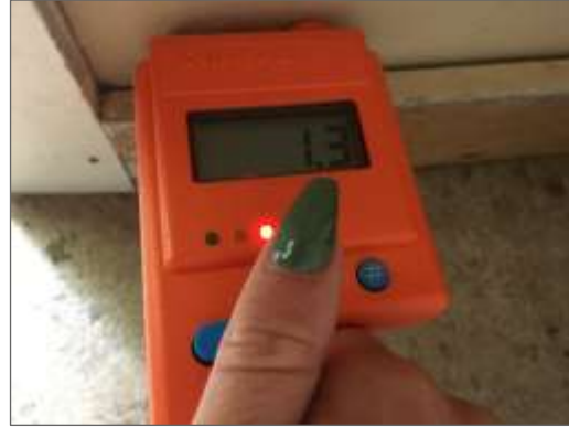
Photo 16 - Wet drywall identified in Living area.
