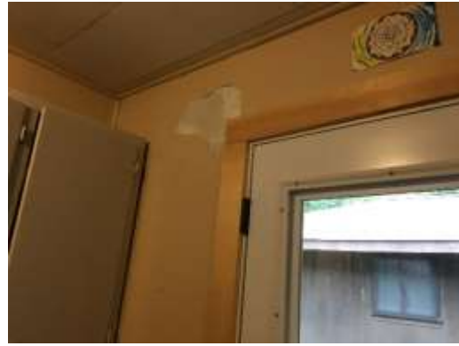
Photo 10 - Water damage to full height of drywall by kitchenette.
