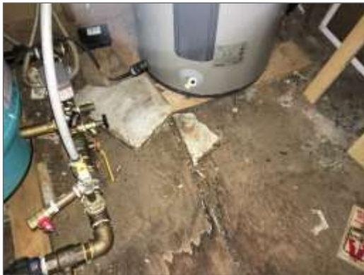
Photo 21 - Water staining on floor and mouse droppings in pump room.
