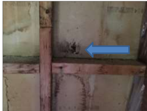
Photo 22 - Organic growth and water staining on drywall in pump room connected to washroom.
