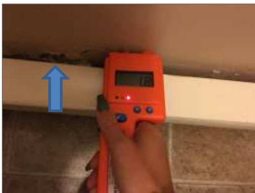
Photo 11 - Water damage identified behind radiator in washroom.
