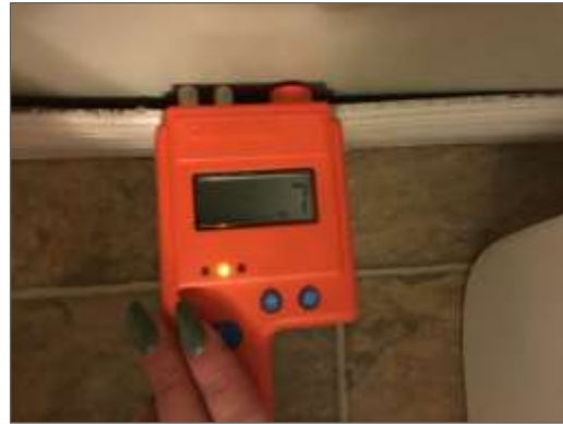
Photo 6 - Wet drywall identified behind toilet in washroom.
