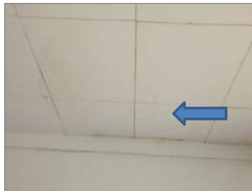
Photo 2 - Faint water staining identified on ceiling tiles.
