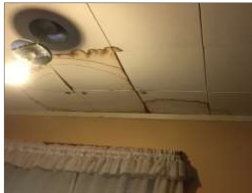
Photo 14 - Typical water staining identified on 1' x 1' tiles in various locations throughout the cabin.
