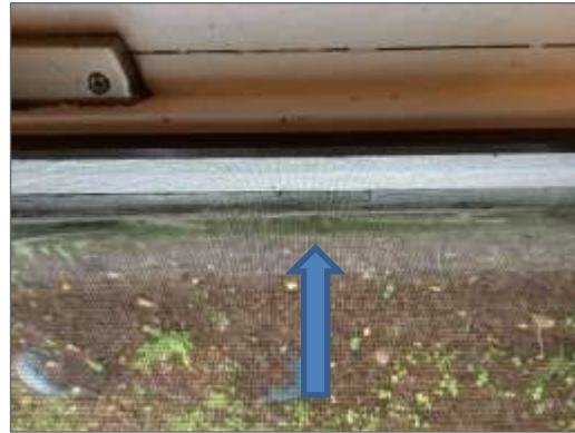
Photo 1B - Organic growth on exterior wood siding below window.
