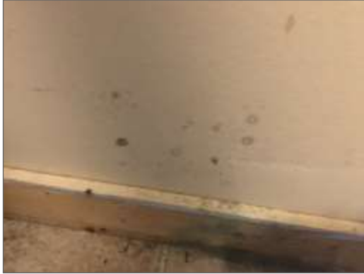
Photo 15 - Mould growth identified on drywall in living area.
