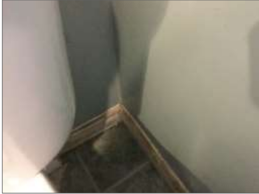
Photo 3 - Previous water damage identified in washroom; drywall is dry.
